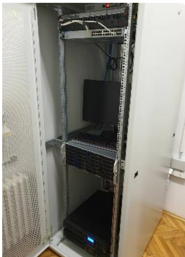
Figure 1. HPC Cluster appearance inside the rack
