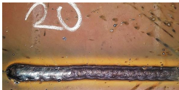
Figure 7 insufficient weaving overlap, weld 20
