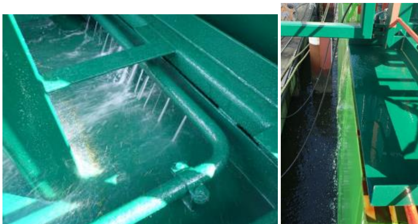
Figure 22 Bunker station in operation
