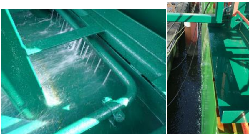
Figure 22 Bunker station in operation
