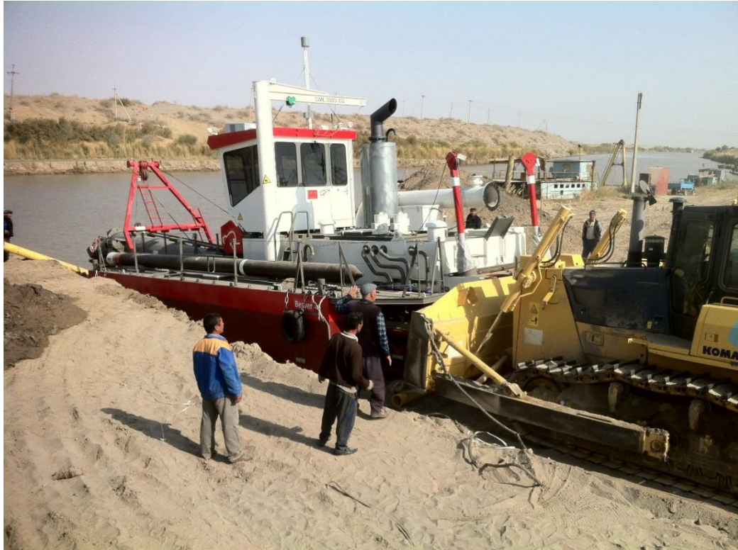
Figure 8 Crawler heavy vehicle used for pushing the IHC Beaver® dredger into the water
