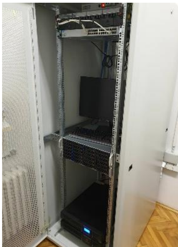
Figure 1. HPC Cluster appearance inside the rack
