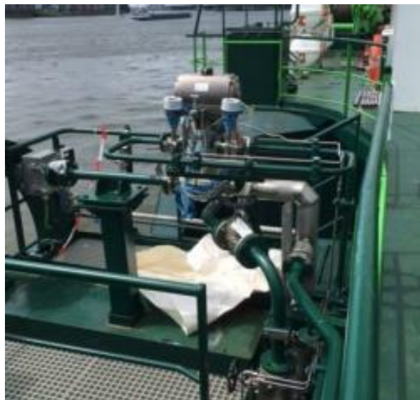
Figure 24 As built situation of bunker station
