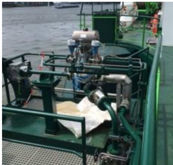
Figure 24 As built situation of bunker station
