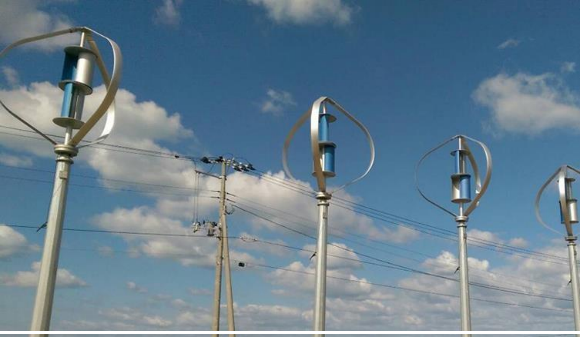
PORTION OF WIND PLANT
